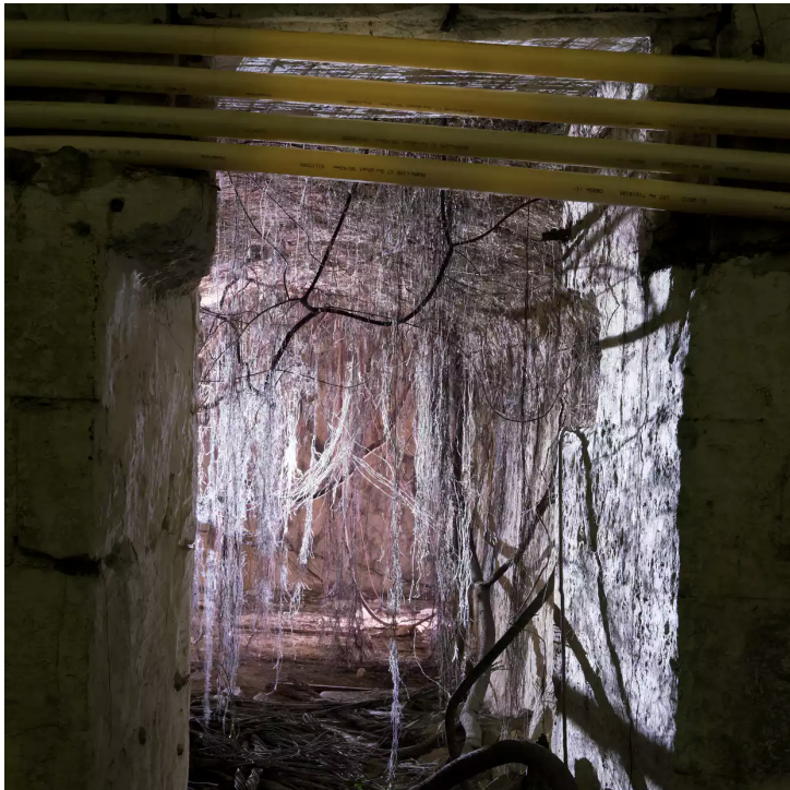
Fibre optic cables stretch over a second world war bunker.
