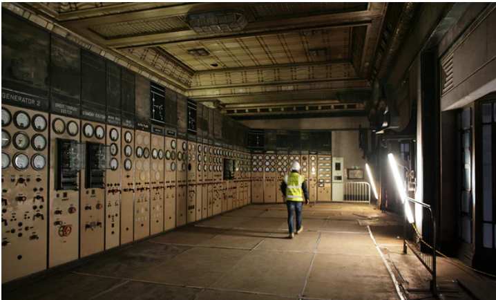
Bradley Garrett explored the control rooms of Battersea power station with what would become the London Consolidation Crew. Photograph: Martin Godwin
