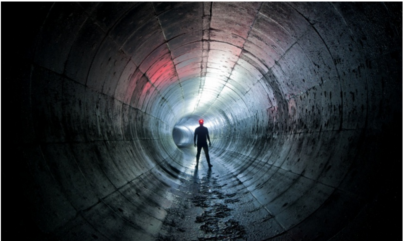
📷 The River Tyburn flows in underground culverts and sewers for its entire length from Hampstead to the Thames
