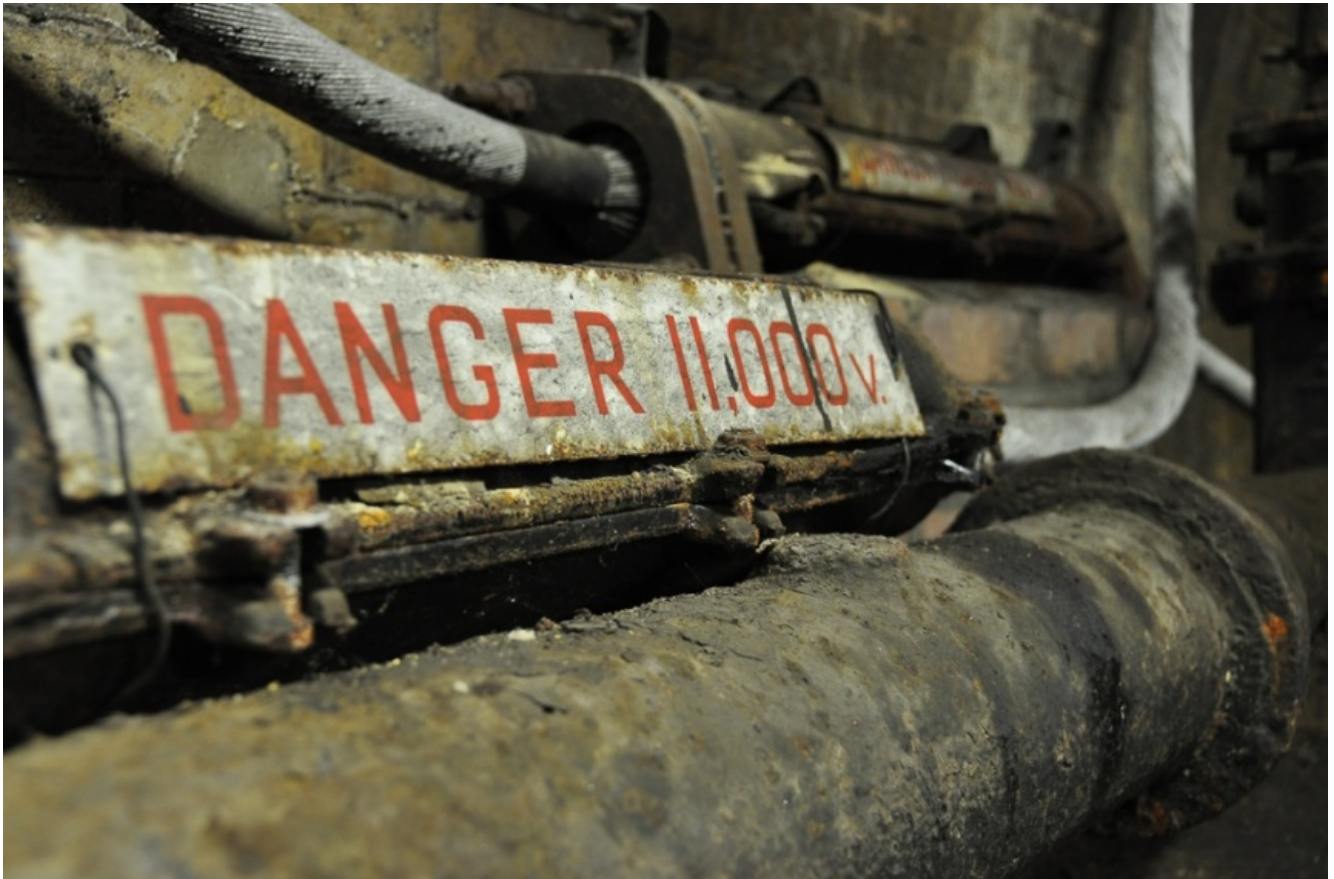
📷 High-voltage electricity cables under central London
